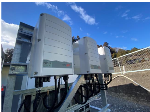
SolarEdge製：SE17.5K-JP3台
